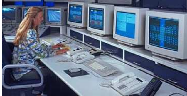
Figure 9.9: Control room of a distributed control system (DCS)
